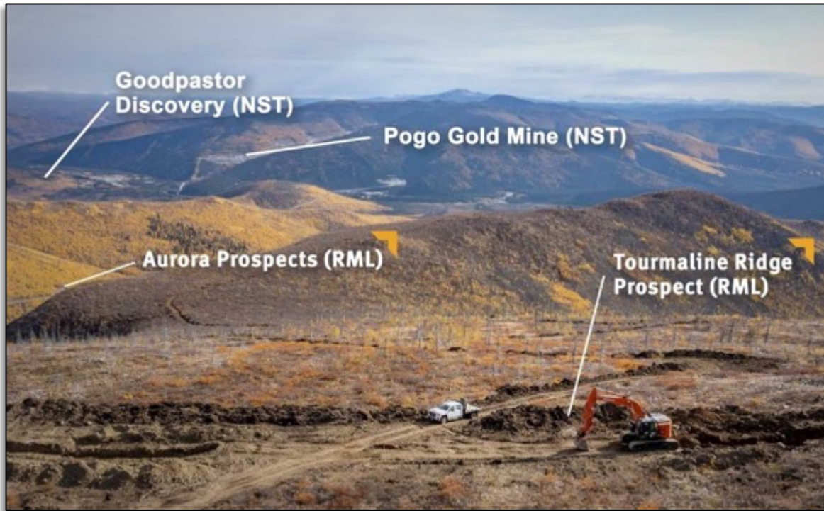
Figure 4 Trenching at Tourmaline Ridge underway September - October 2021, with the Pogo Gold Mine in the background.
